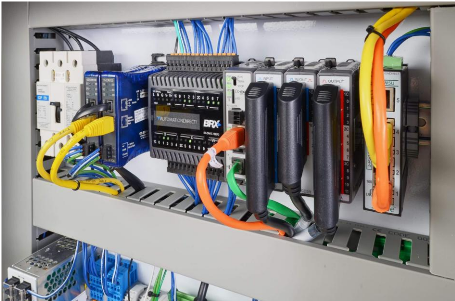
Networked Industrial Automation (Devices)
